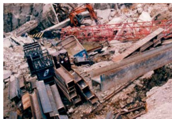
LEFT: A bird's eye view of the tragic collapse of Nicoll Highway.
