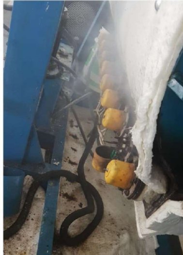
Figure 25: Photograph taken by Marimuthu on 24 February 2021 at 1113hrs showing that the wiring of the damaged heater #2 had been taped together with green tape
