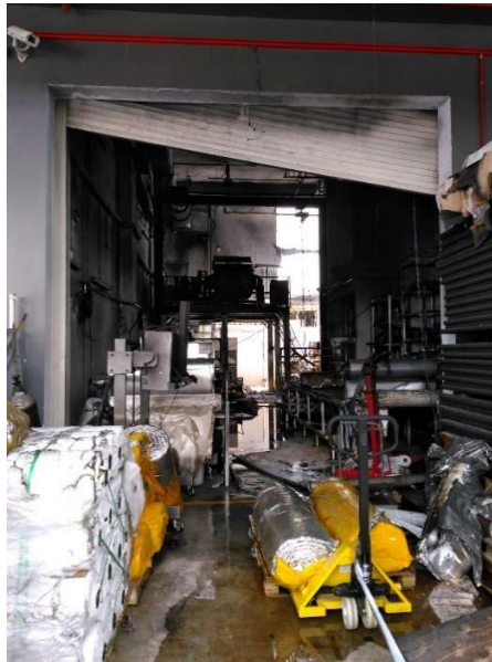
Figure 28: Damaged front shutters of the worksite
