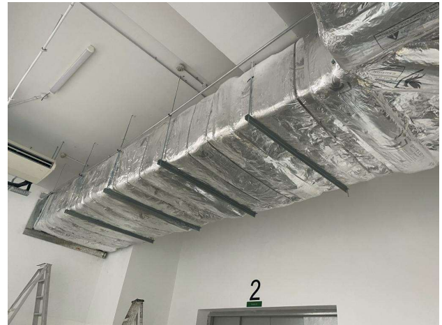
Figure 1: Fire wrap on ducting
