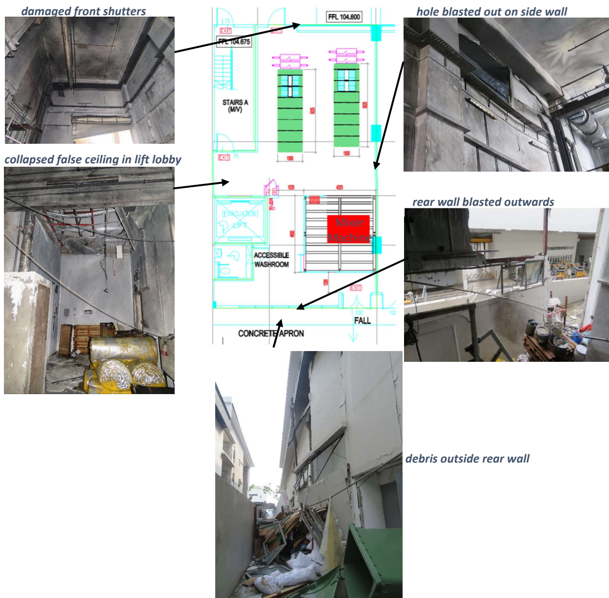
Figure 27: General damage within the worksite
