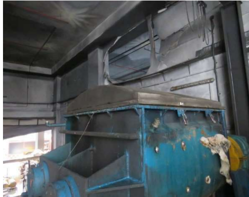
Figure 32: Hole at the top of side wall
