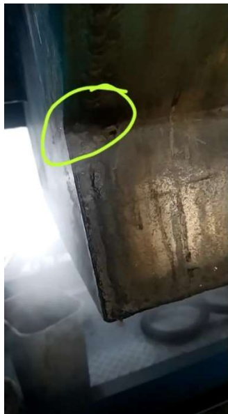
Figure 16: Screenshot from video of 12 October 2020 showing oil leak and smoke, green circle inherent in video
