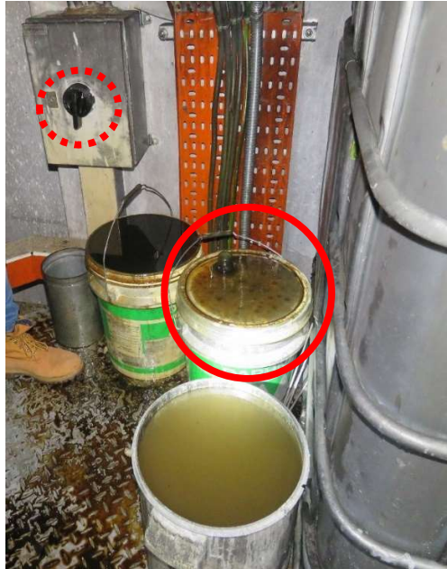
Figure 42: Covered bucket (circled in red) and mixer machine's isolator in the "ON" position (dotted circle in red)
