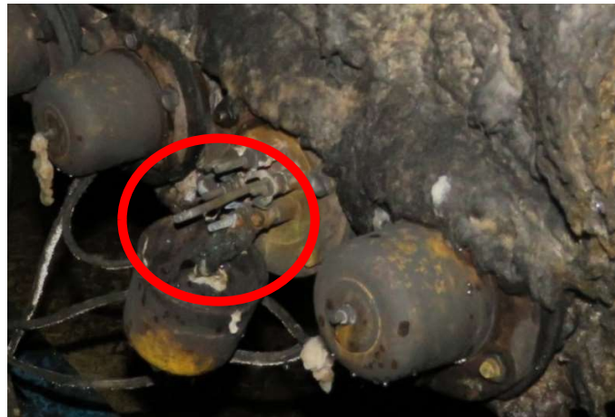
Figure 46: Green tape found on wires connected to two terminal connections of heater #2
