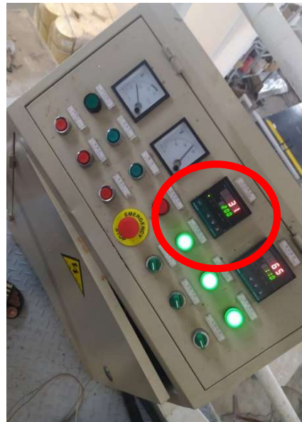
Figure 17: Safety interlock temperature setting at 200°C on 12 October 2020, green digits within red circle
