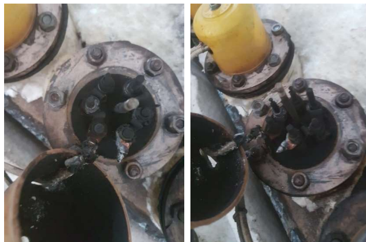
Figure 23: One of the cables on heater #2 had snapped, likely due to the earlier fire
