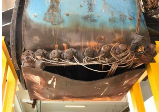
Figure 53: Bulging deformation, indicative of overpressure release from inside out
