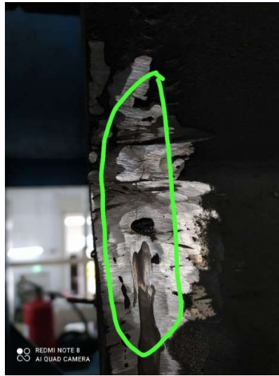
Figure 21: Grinding revealed a hairline crack on front left of machine, green circle inherent in picture
