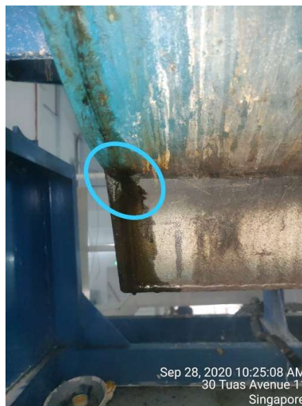
Figure 14: First oil leak on jacket, blue circle inherent in Imam’s photograph
