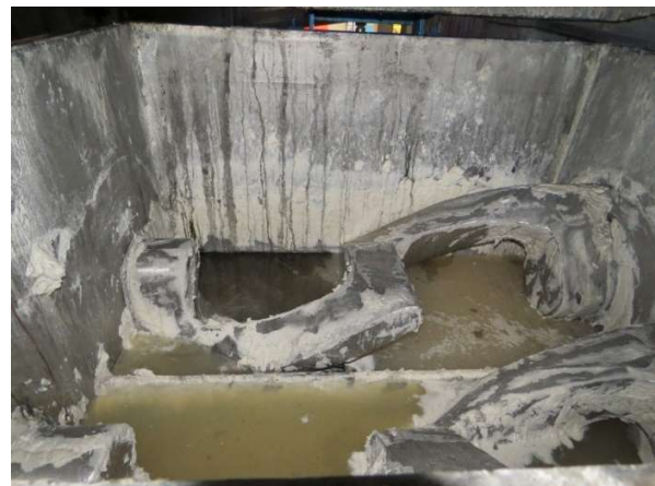
Figure 45: Inside of the mixing chamber
