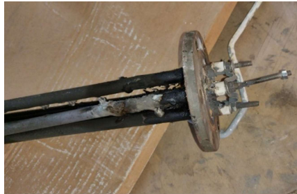
Figure 50: Photo showing replaced heater #1 (taken from Chua's phone pre-explosion)
