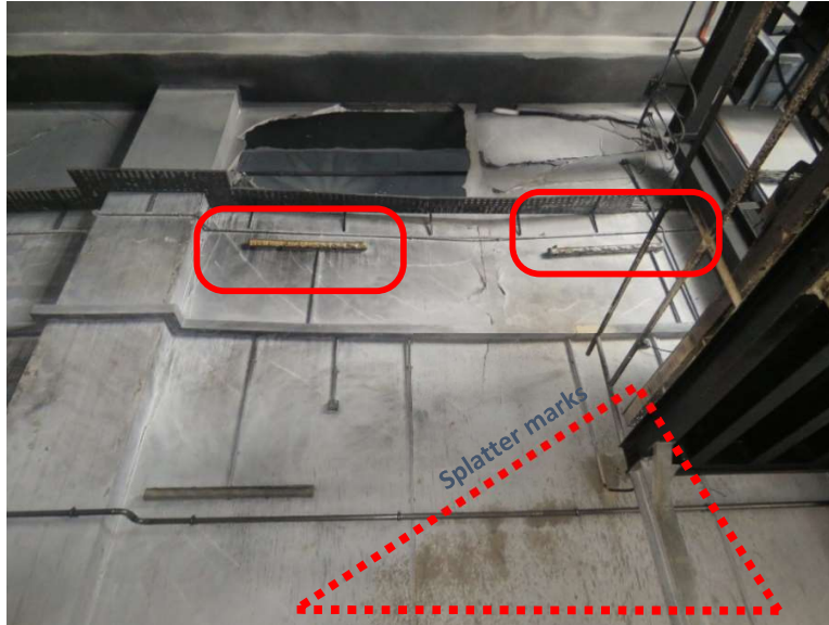
Figure 30: Photo showing the damaged light fixtures and splatter marks from platform
