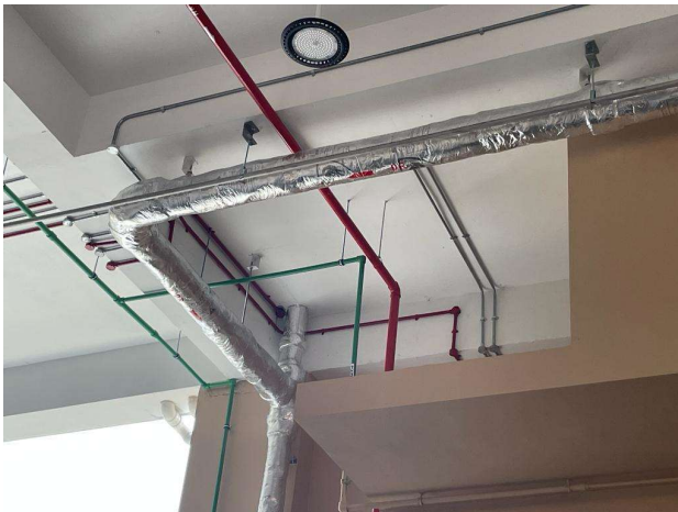
Figure 1: Fire wrap on pipes
