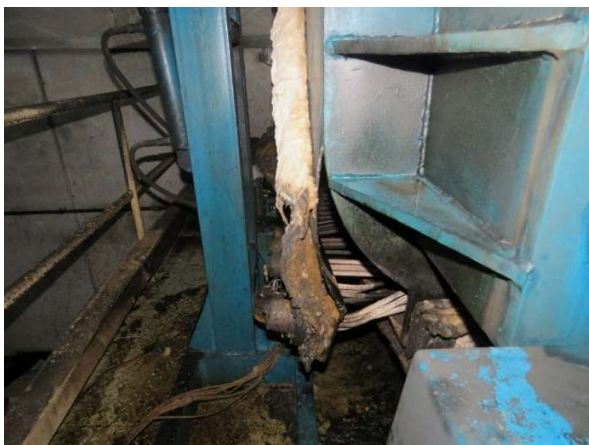
Figure 37: Deformed heating elements seen through the rupture on the oil jacket, rear of machine
