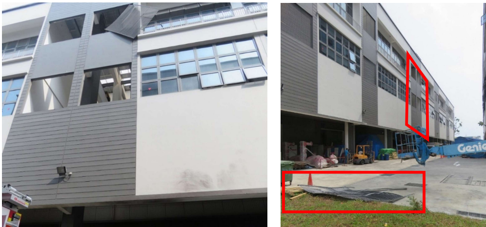
Figure 33: Photos showing the dislodged louvre panels
