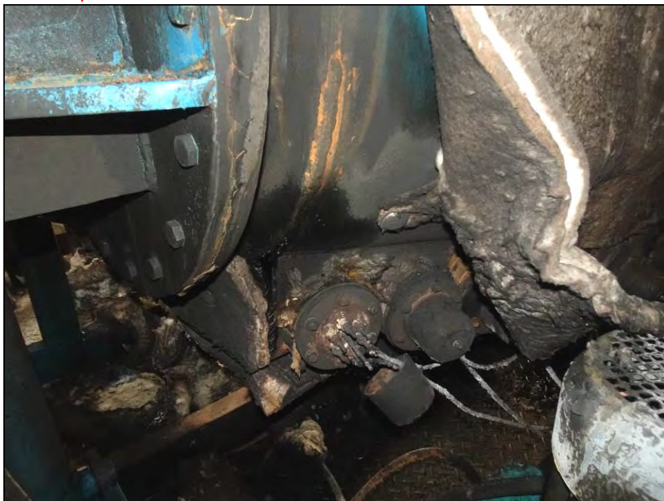
Tearing along the weld joint of the oil jacket around the heater
