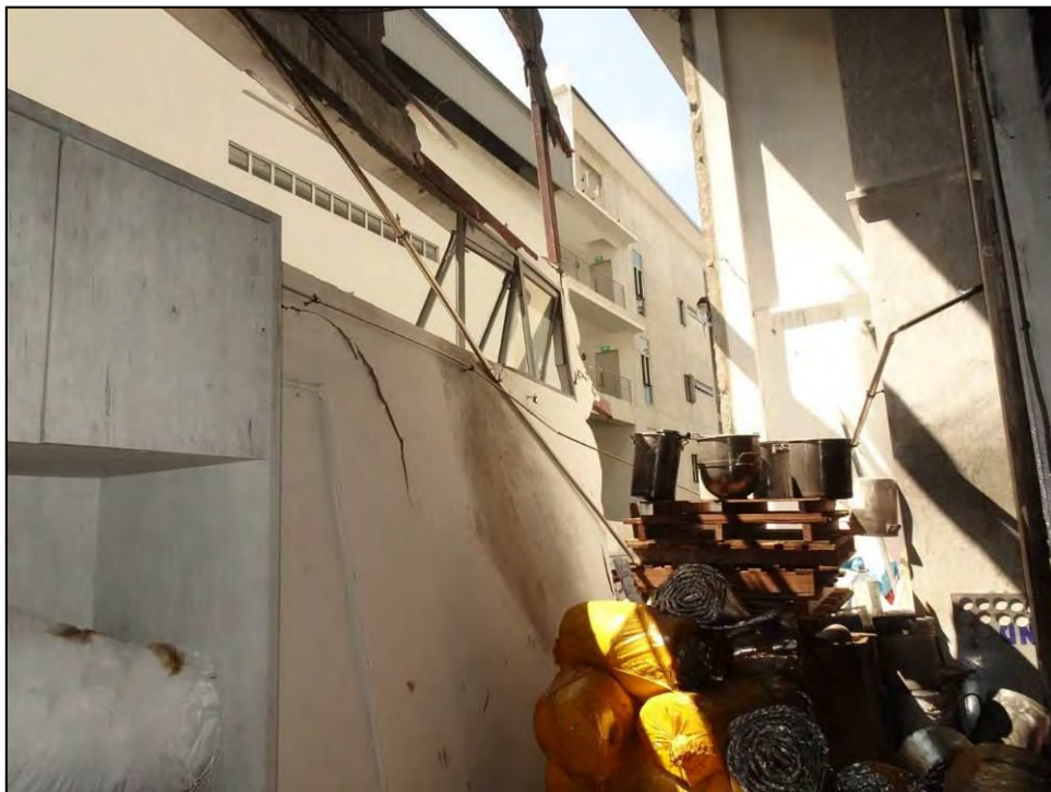
Punctured wall at the rear end of the unit
