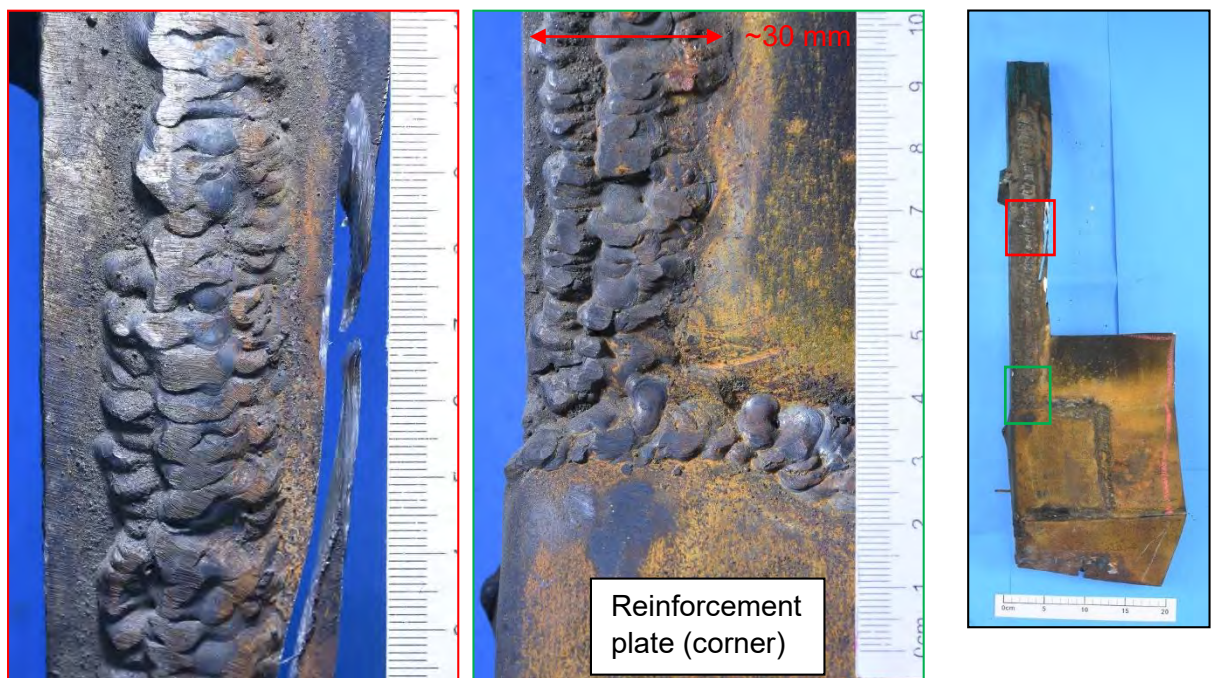
Figure 43: Close up view of side weld. The face width of the weld increases towards the bottom and reinforcement corner plate. The face width was up to about 30 mm.
