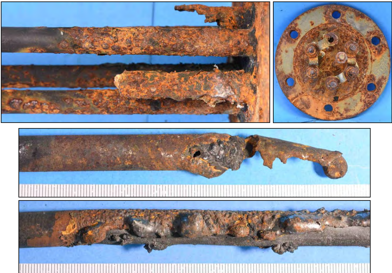
Figure 114: One of the coil had broken off from the heater. The metal tube had deformed and melted off around the breakage location as evidenced by the bulbous and droplet-like shape of the metal.
