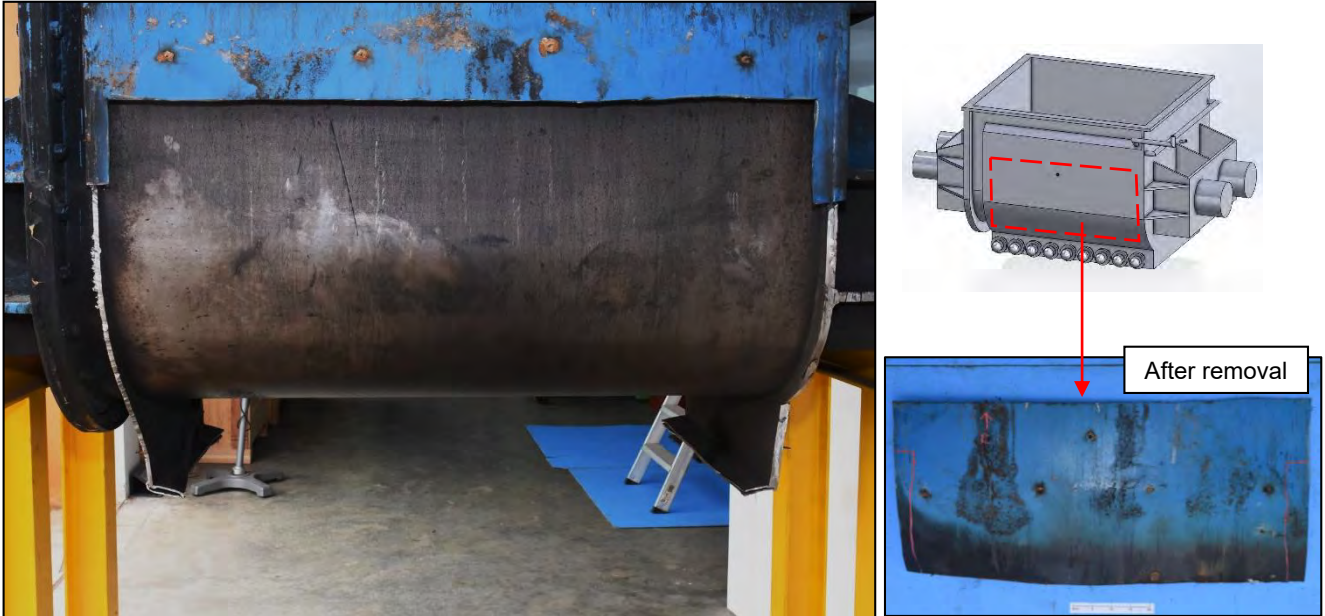
Figure 59: Internal condition of the oil jacket from the rear side. The internal surface was generally covered by black soot.
