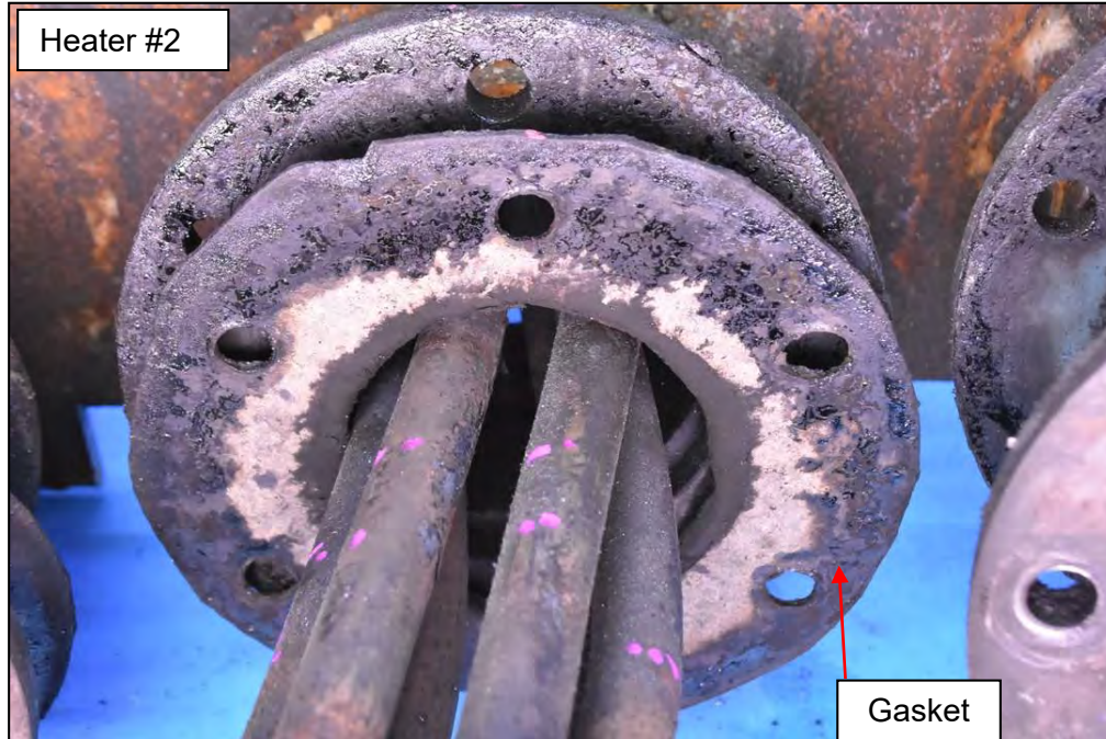
Figure 87: Due to the severe deformation, heaters #1, #2 and #3 cannot be removed without cutting the metal tubes. The gaskets were generally brittle with some parts still adhering to the flanges' surface.
