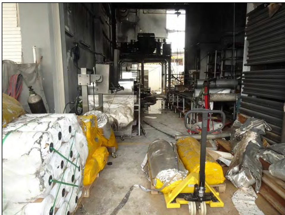
Front end of the incident unit
