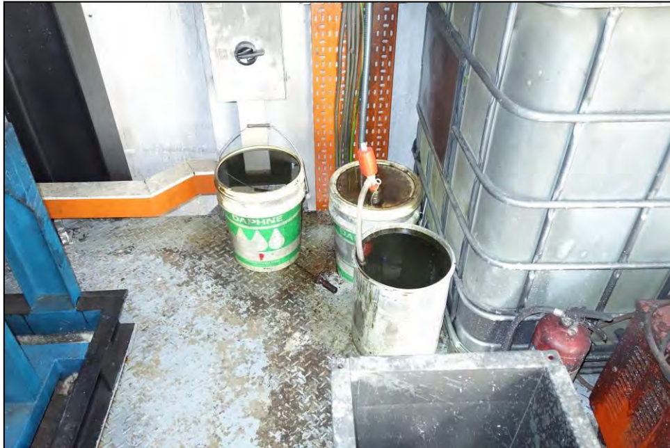
Oil pails on Platform floor
