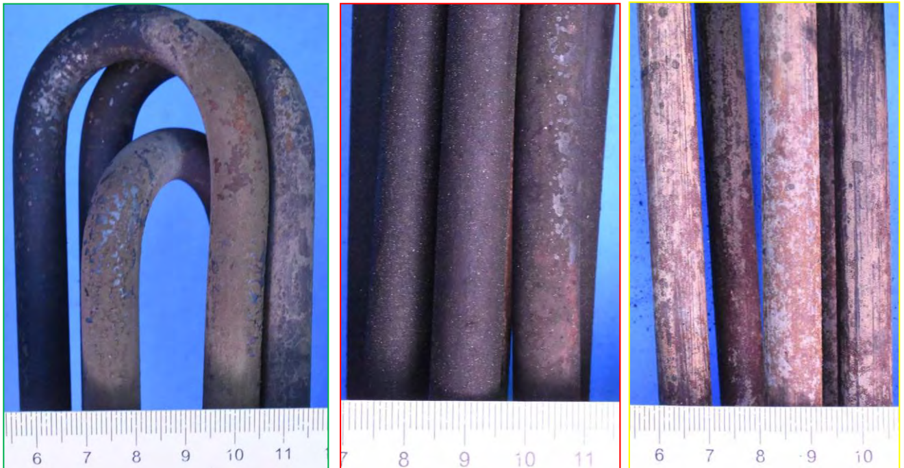
Figure 86: Signs of corrosion and peeling of coating were observed at various parts of the metal tubes.
