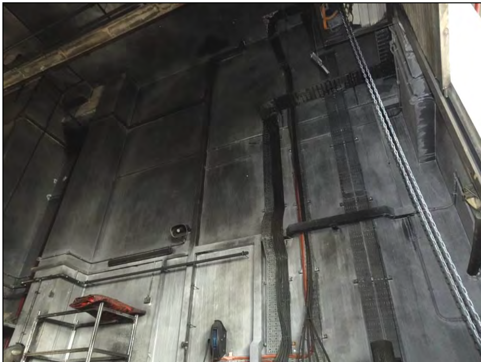
Charred walls towards the front of the unit
