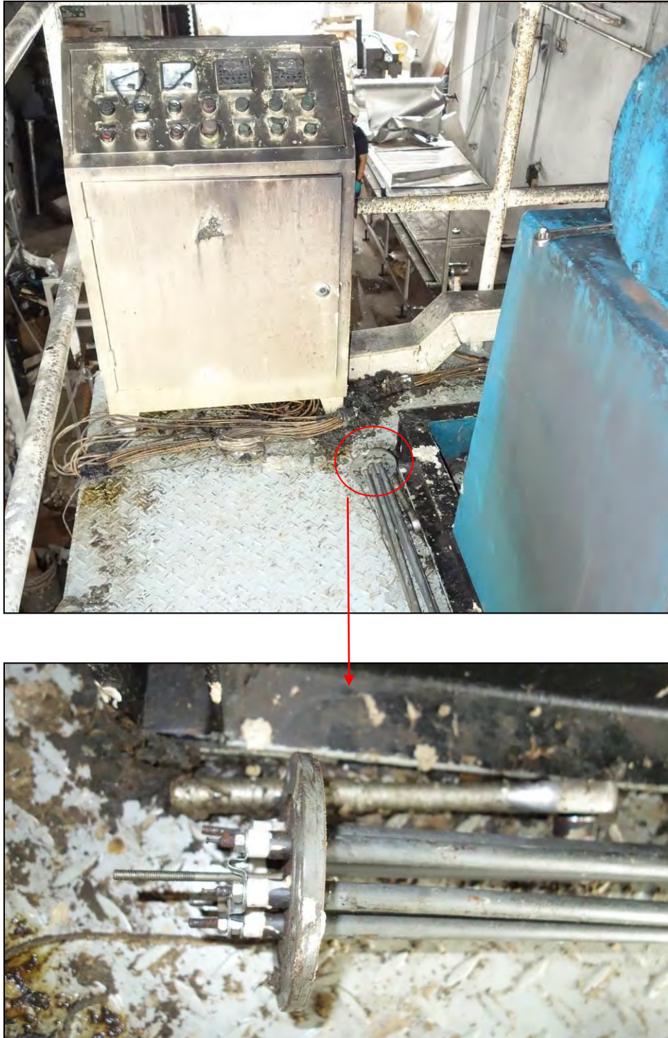
Electrical panel box (top, left) and new heater (circled)
