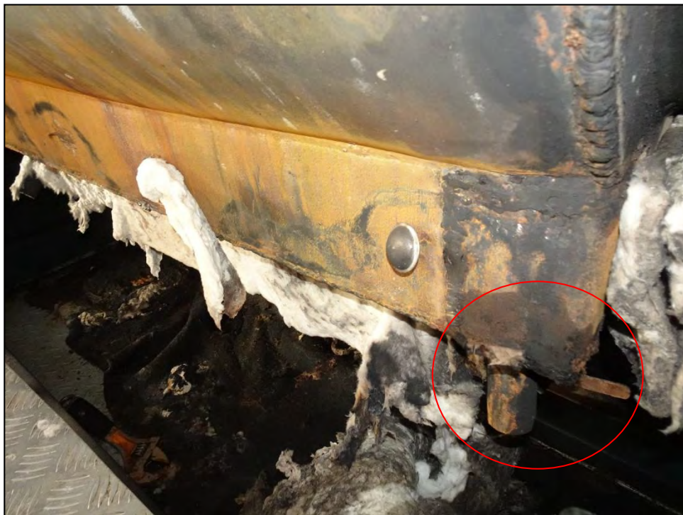
Drain port for oil jacket (circled)
