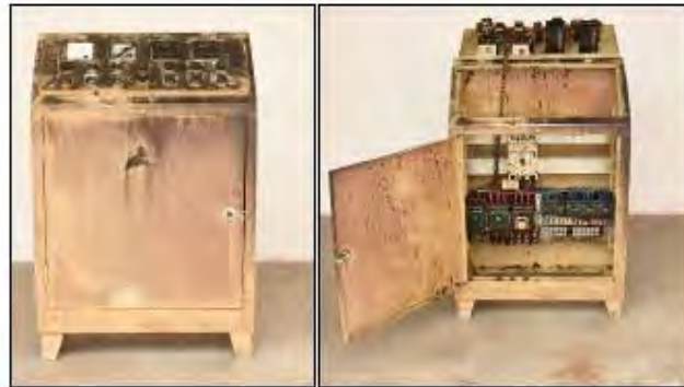
As-received condition of local control panel.
