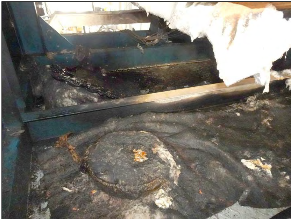
Charred insulation wools on the Platform floor under the oil jacket
