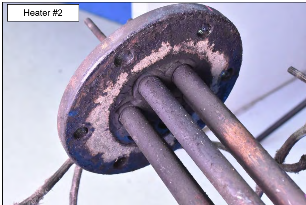
Figure 88: Heater flange condition from the side adhering to the gasket.
