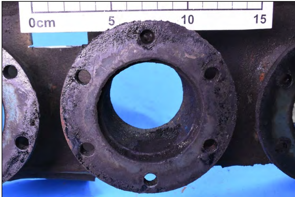
Figure 89: The rest of the heaters were removed, revealing generally similar flange condition. Oil residue were present inside.
