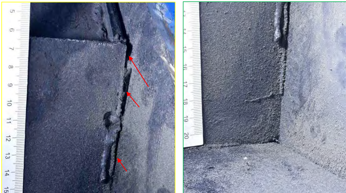
Figure 49: Close up view of the corner from inside the oil jacket. Gaps were observed between the walls (indicated with red arrows). The gap narrowed and stopped towards the bottom corner.
