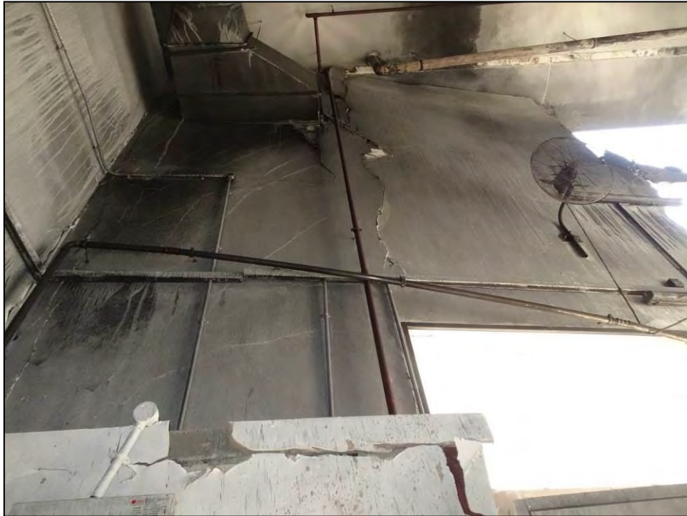
Cracked wall at the rear end of the unit
