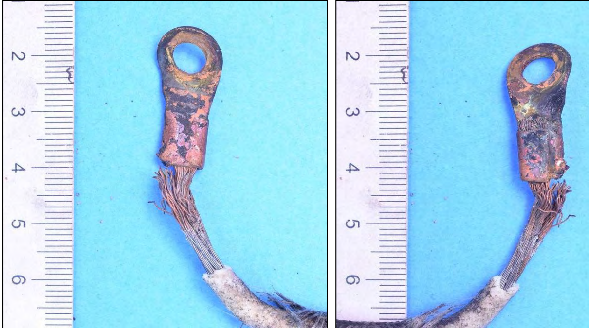
Figure 131: Wire and lug of heater #2, terminal 3.
