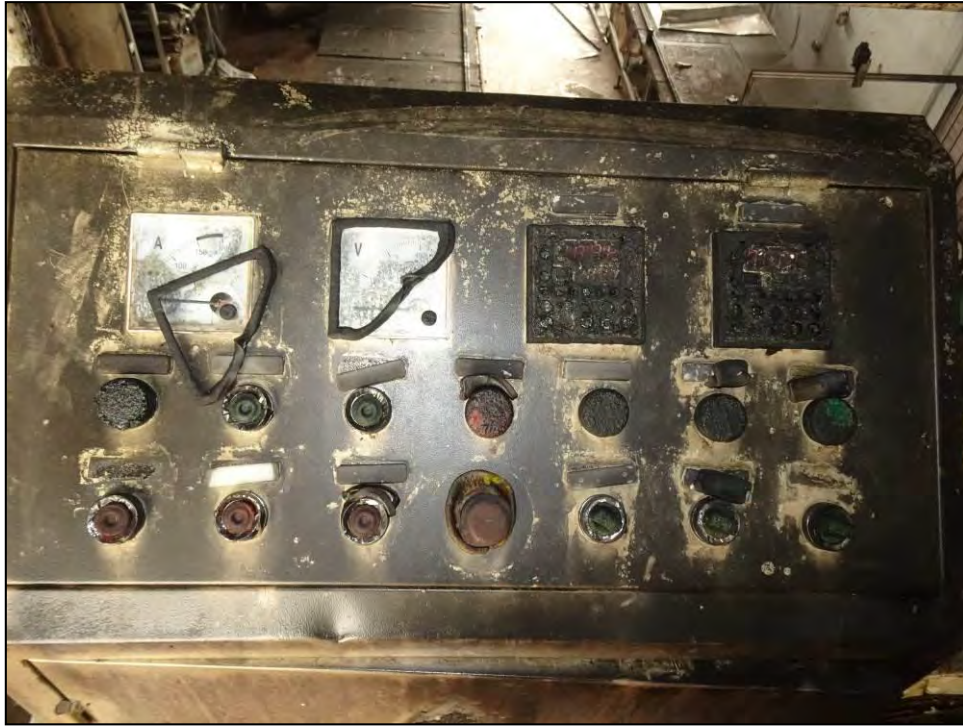
Partially melted electrical switches and buttons
