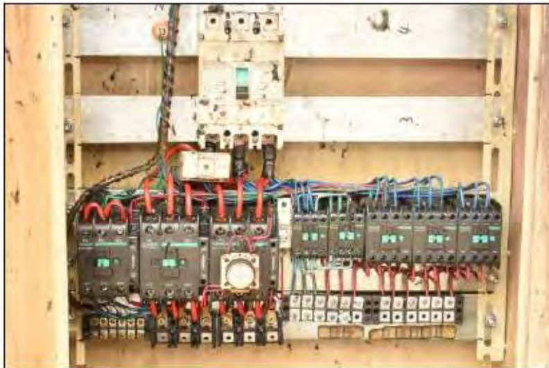
View of components from inside the LCP.
