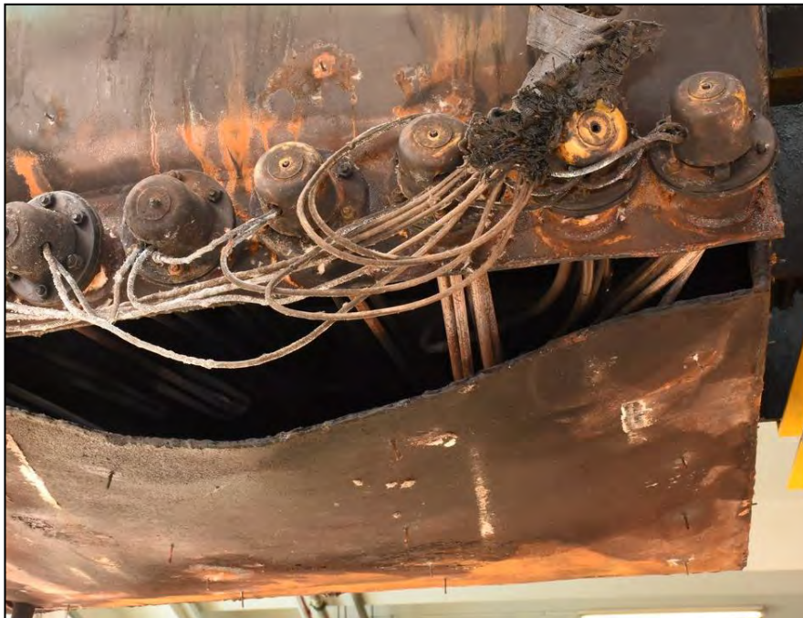
Figure 30: As-received condition of the Mixer Machine as seen from the rear bottom.
